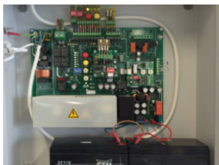
Photo 12. RWZ 4d smoke extraction system control panel.
