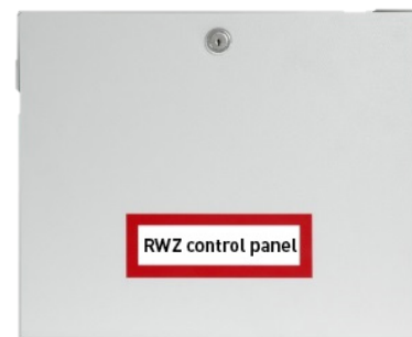
Photo 11. RWZ 1b smoke extraction system control panel.
