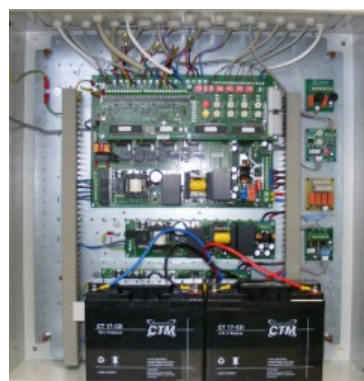
Photo 13. RWZ 5e smoke extraction system control panel.
